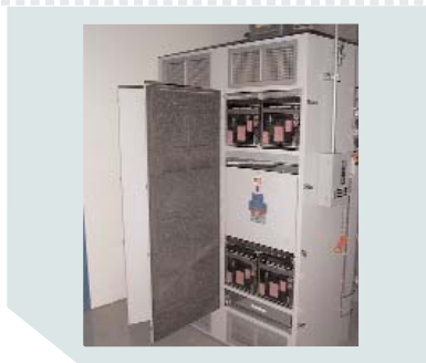
PURAFIL POSITIVE PRESSURIZATION UNIT IN ROLL GRIND ROOM
